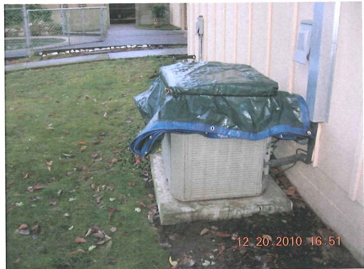
HEAT PUMP ON CONCRETE PAD
