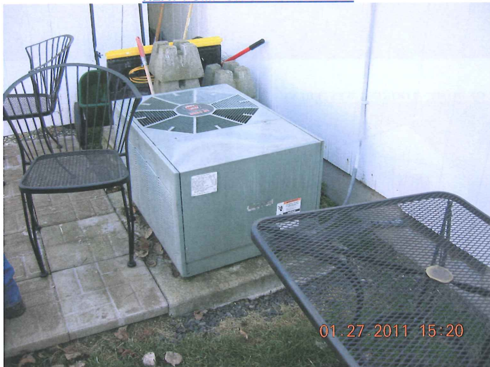
HEAT PUMP ON CONCRETE PAD
