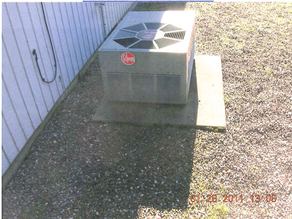
HEAT PUMP ON CONCRETE PAD
