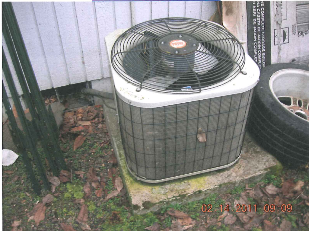
HEAT PUMP ON CONCRETE PAD
