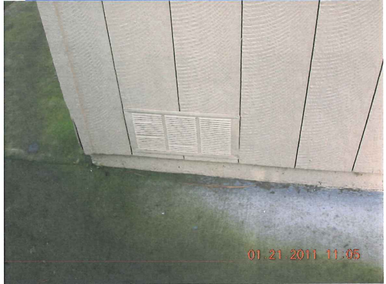
FOUNDATION VENT WITH A LOUVERED COVER (2)
