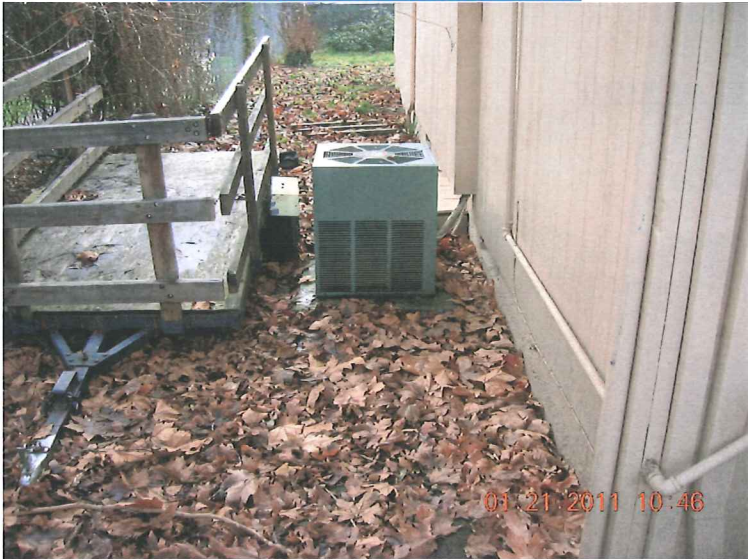
HEAT PUMP ON CONCRETE PAD
