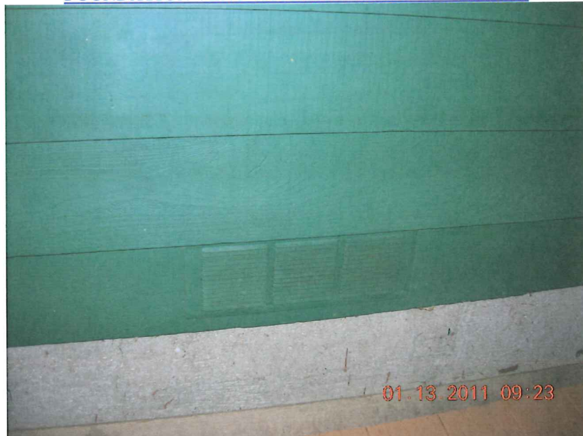
FOUNDATION VENT WITH LOUVERED COVERS (13)
