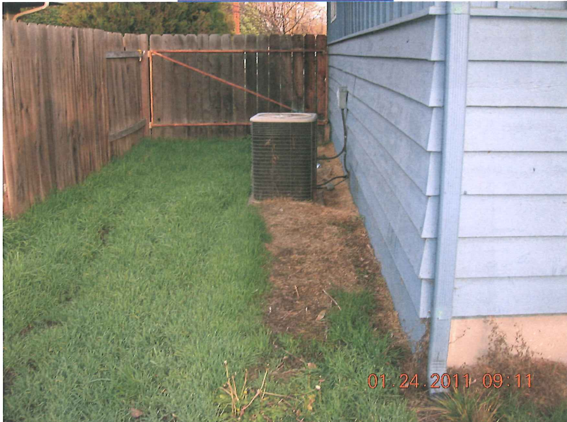
HEAT PUMP ON CONCRETE PAD
