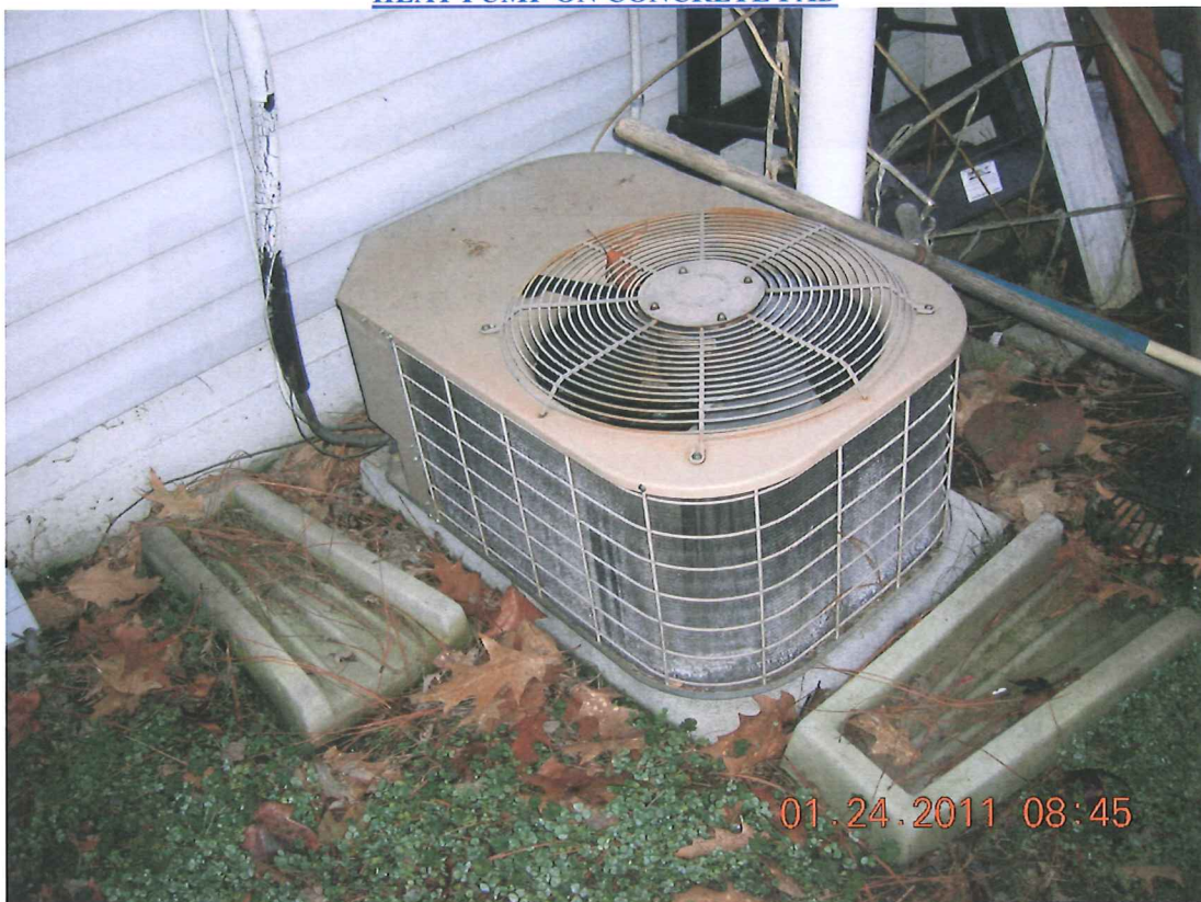
HEAT PUMP ON CONCRETE PAD
