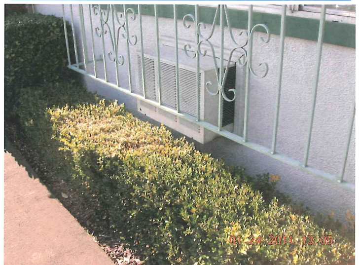
ELEVATED WALL-MOUNT AIR CONDITIONING UNIT
