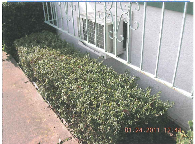
ELEVATED WALL-MOUNT AIR CONDITIONING UNIT
