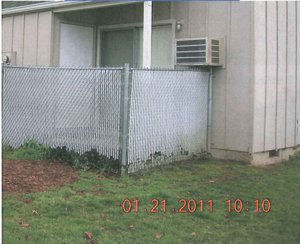
WALL MOUNTED AIR CONDITIONING UNIT
