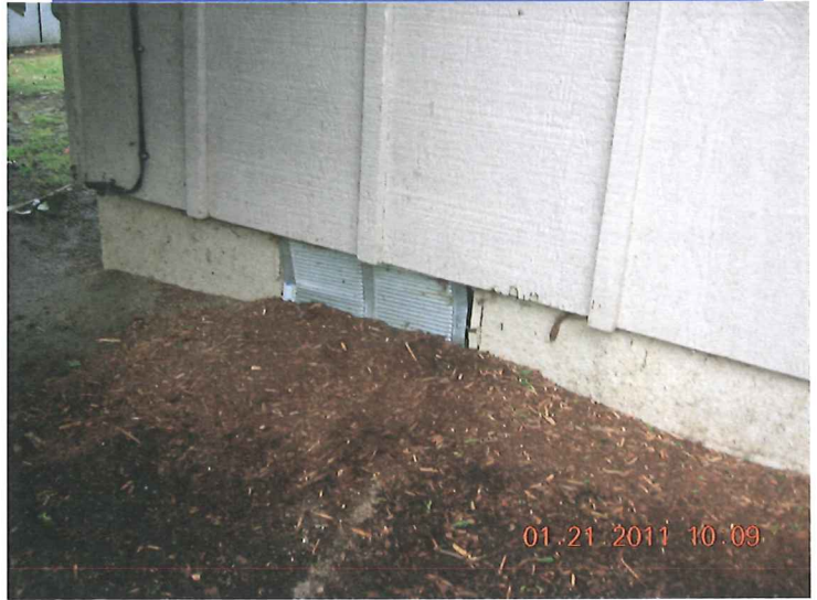
FOUNDATION VENT WITH LOUVERED COVER (1)
