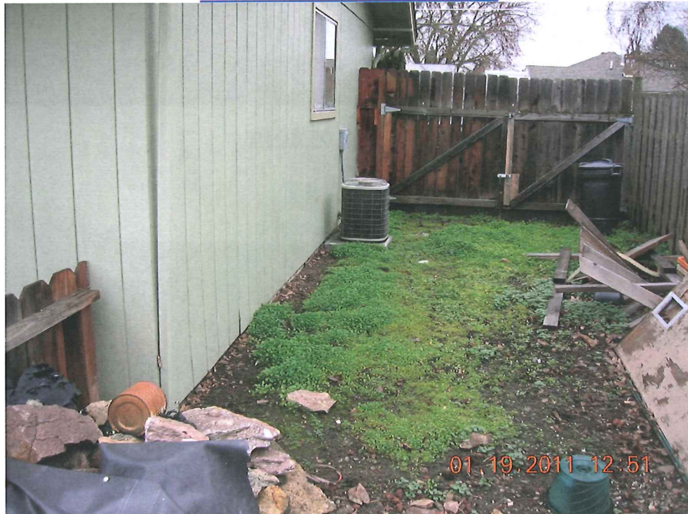
HEAT PUMP ON CONCRETE PAD
