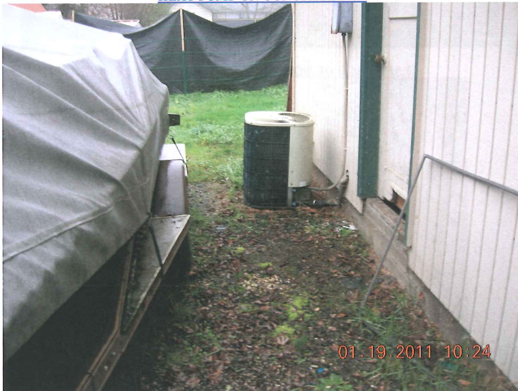
HEAT PUMP ON CONCRETE PAD
