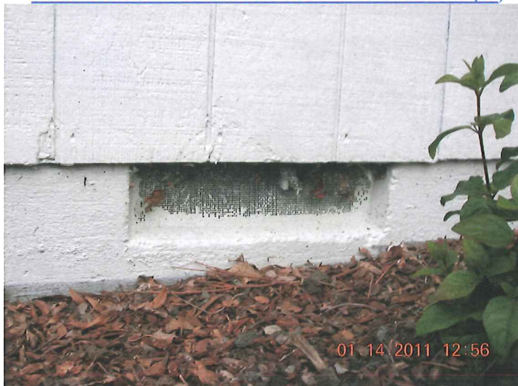
FOUNDATION VENT WITH SCREEN COVERING (11)
