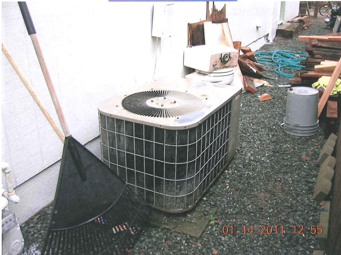
HEAT PUMP ON CONCRETE PAD
