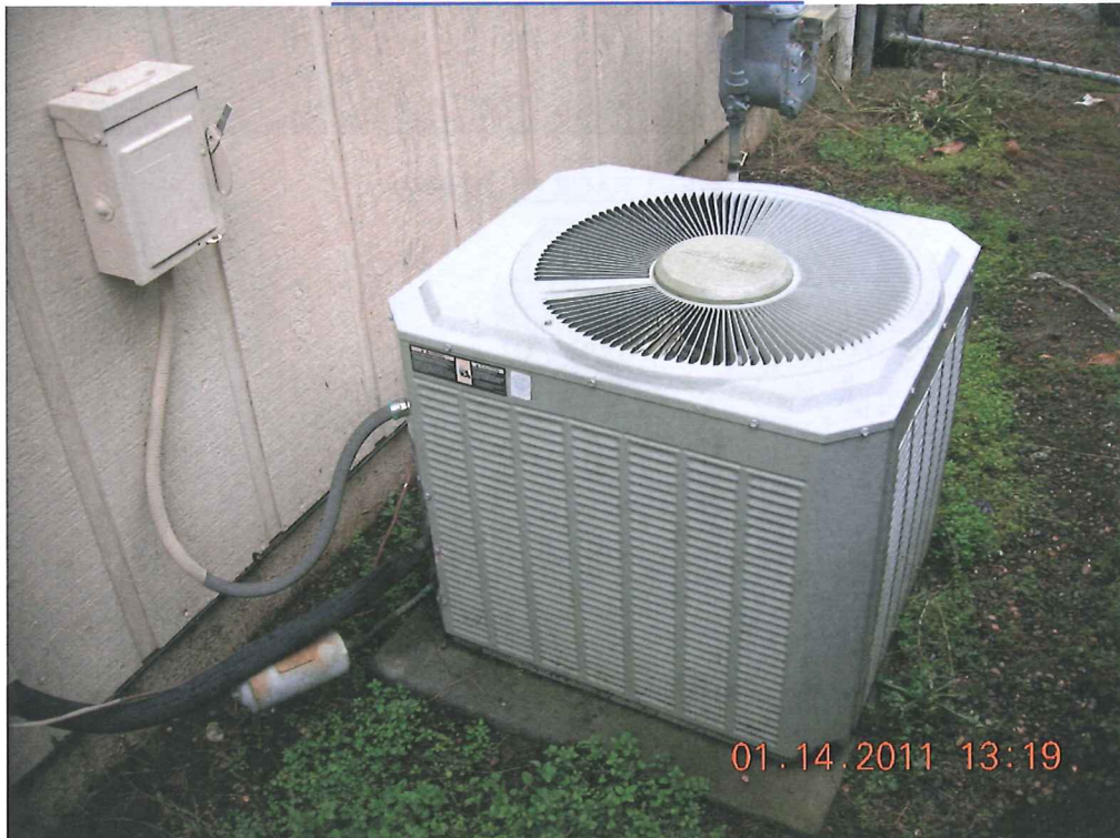
HEAT PUMP ON CONCRETE PAD
