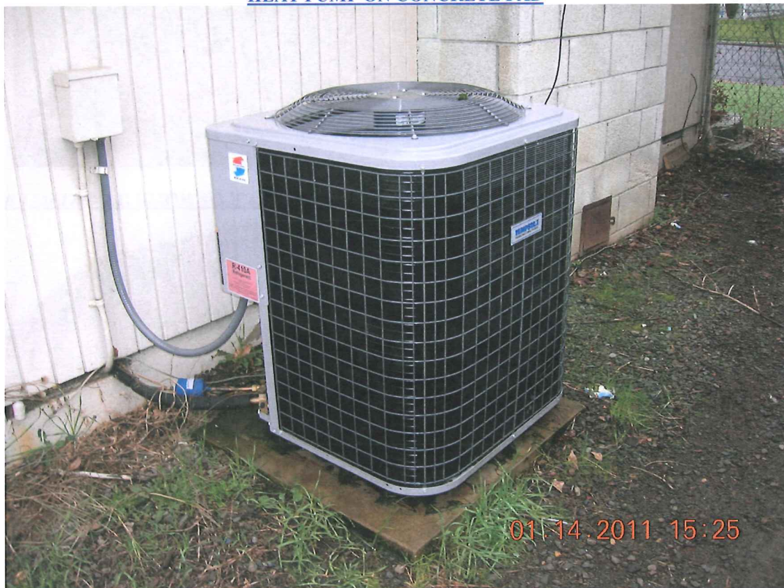
HEAT PUMP ON CONCRETE PAD
