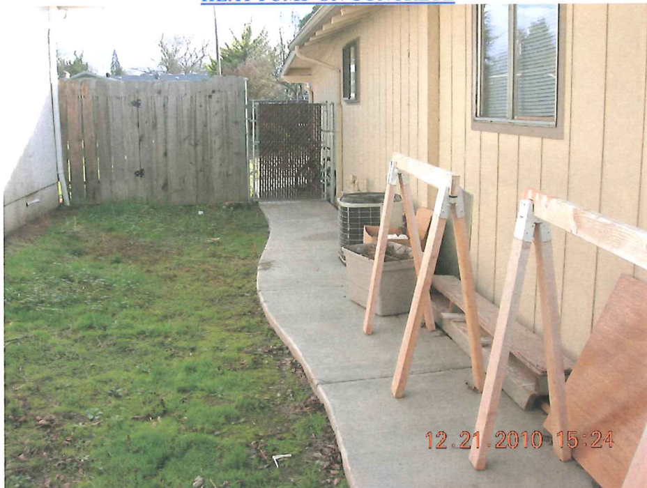
HEAT PUMP ON CONCRETE
