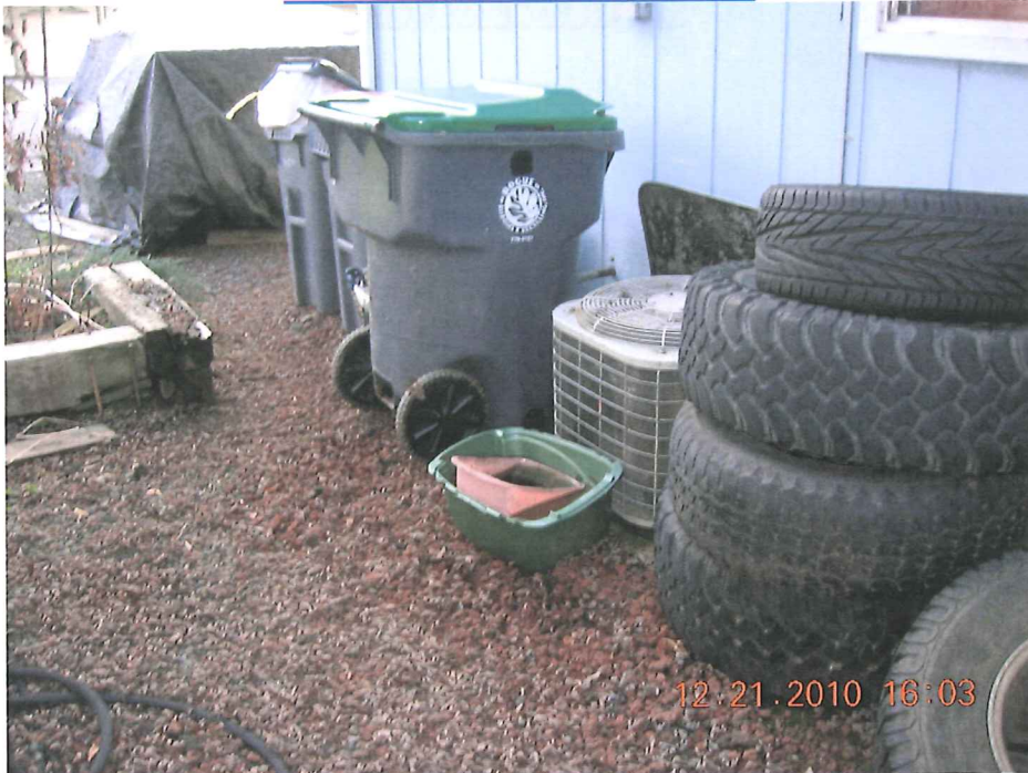
HEAT PUMP ON CONCRETE PAD
