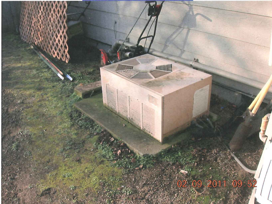
HEAT PUMP ON CONCRETE PAD
