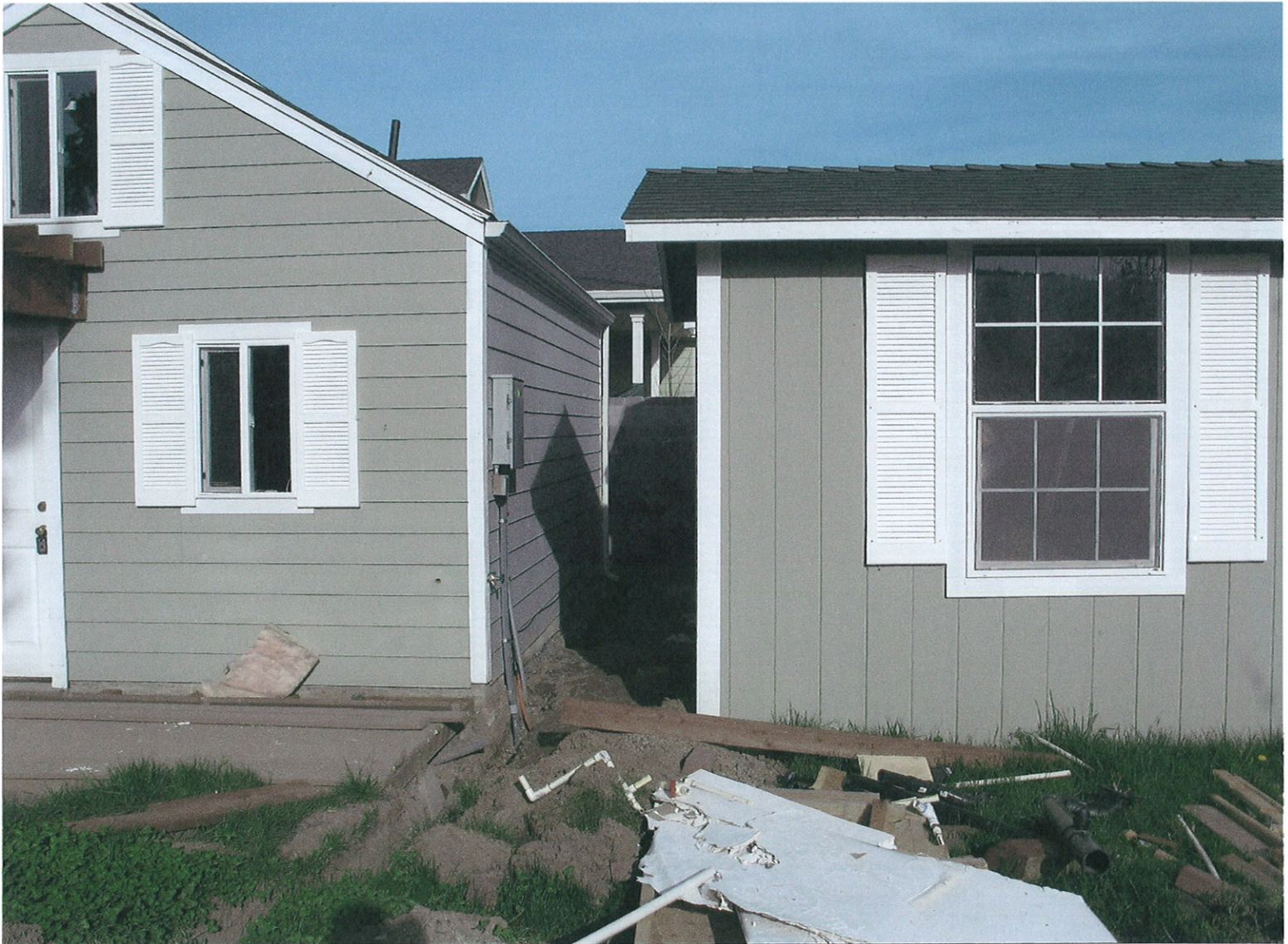
Southwest side of apartment next to shed. Underground power connection. Jackson Creek is to the south (right). Date taken March 30, 2007.
