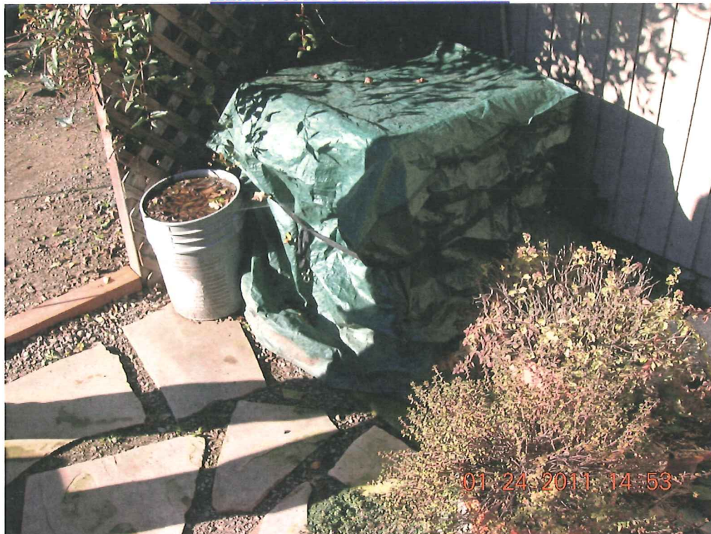
HEAT PUMP ON CONCRETE PAD
