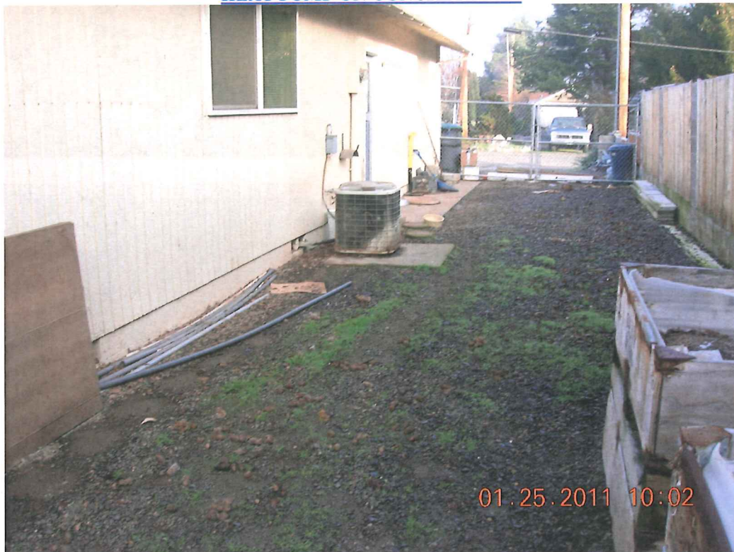
HEAT PUMP ON CONCRETE PAD
