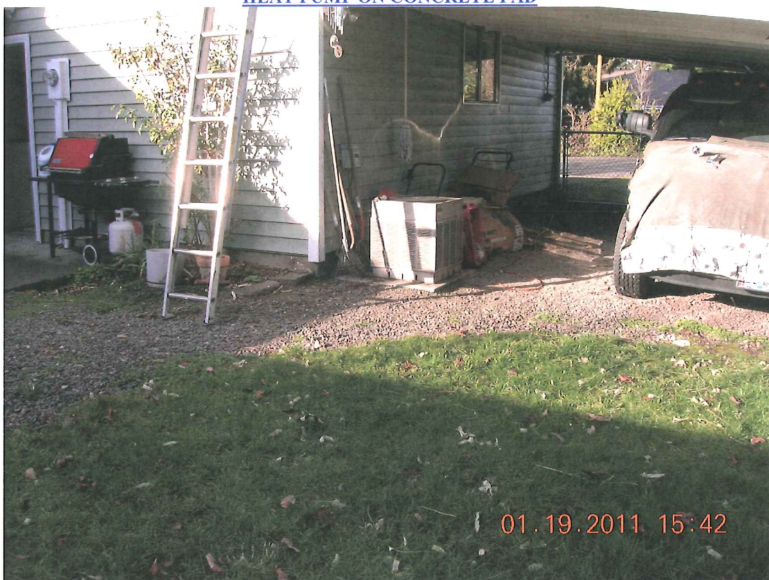
HEAT PUMP ON CONCRETE PAD
