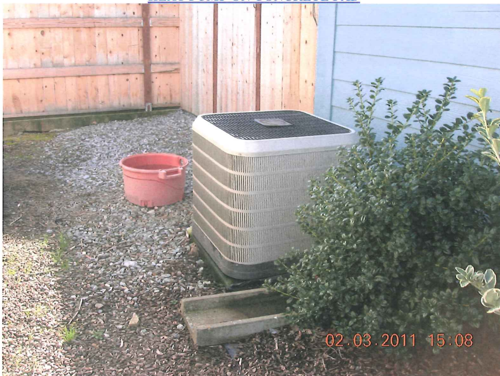
HEAT PUMP ON CONCRETE PAD
