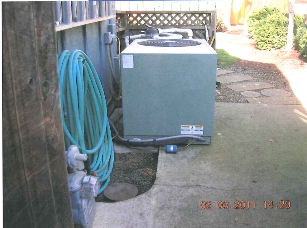
HEAT PUMP ON CONCRETE PAD
