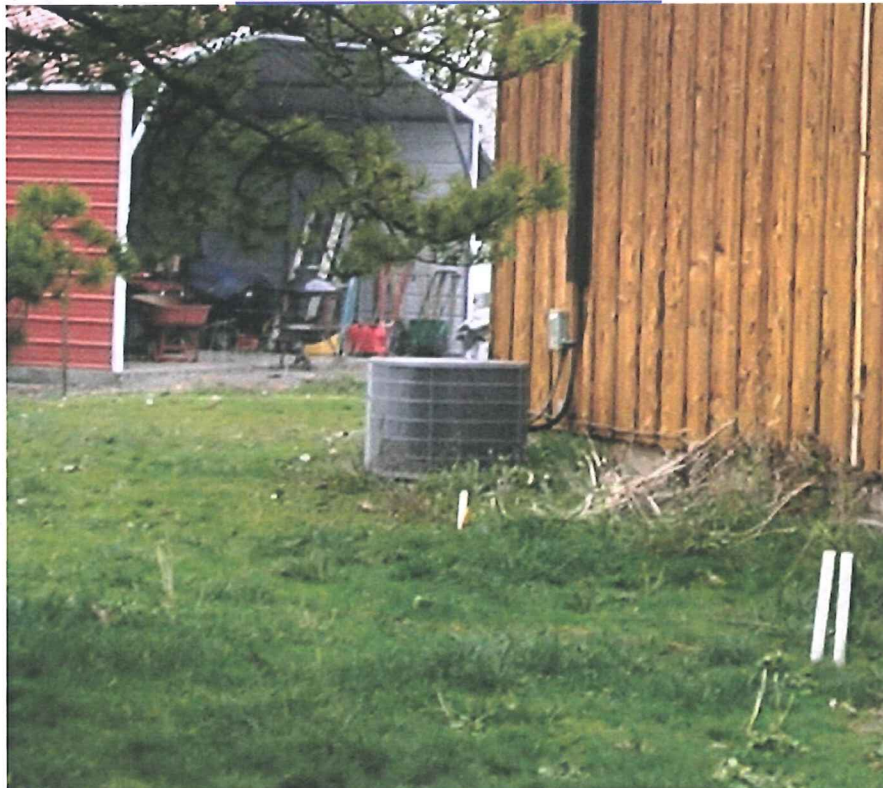
HEAT PUMP ON CONCRETE PAD
