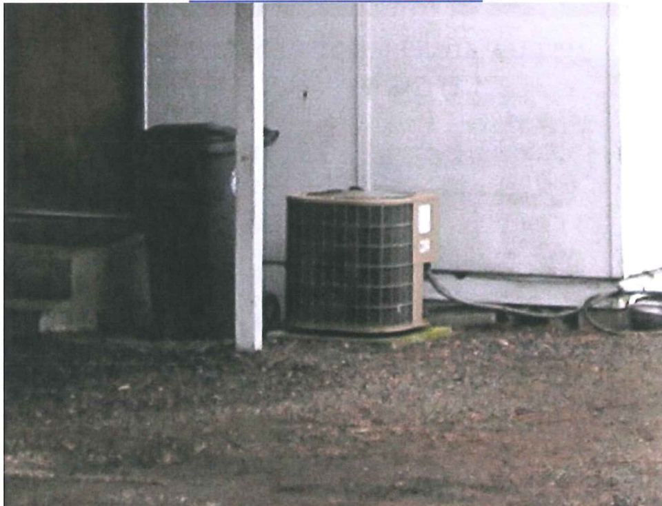
HEAT PUMP ON CONCRETE PAD
