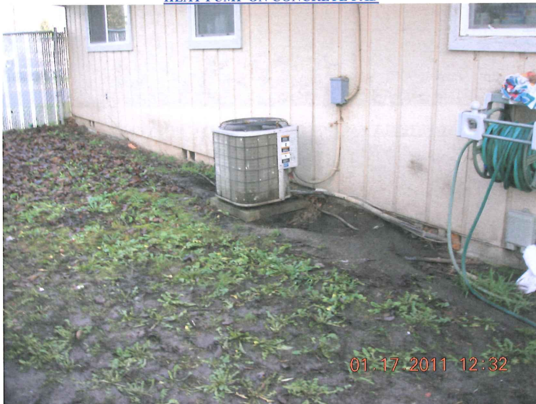
HEAT PUMP ON CONCRETE PAD
