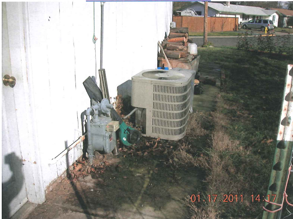
HEAT PUMP ON CONCRETE PAD
