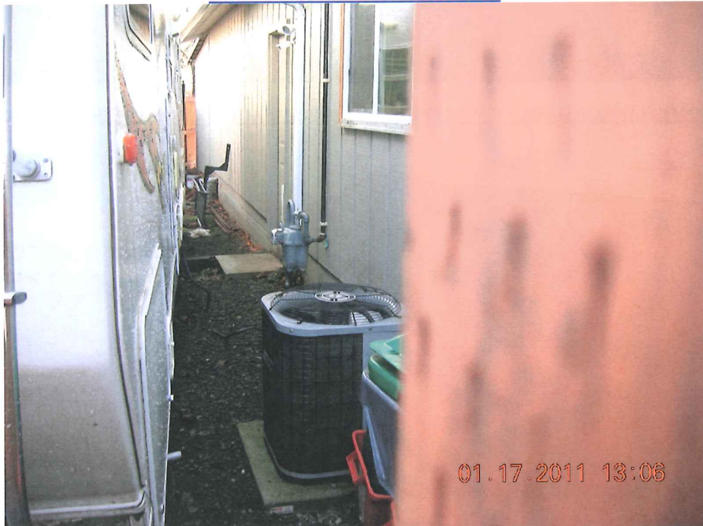
HEAT PUMP ON CONCRETE PAD
