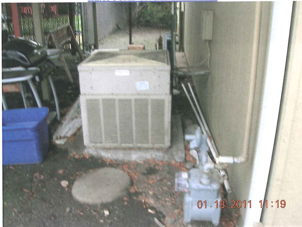
HEAT PUMP ON CONCRETE PAD
