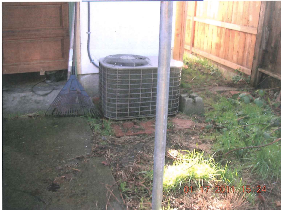
HEAT PUMP ON CONCRETE PAD
