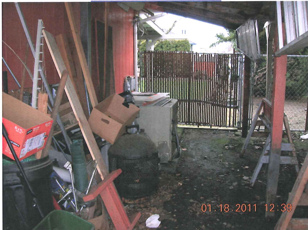
HEAT PUMP ON CONCRETE PAD
