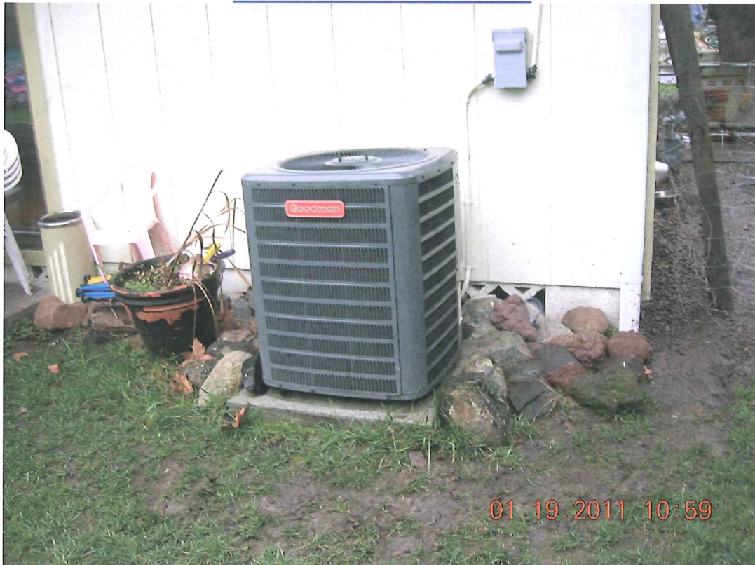
HEAT PUMP ON CONCRETE PAD
