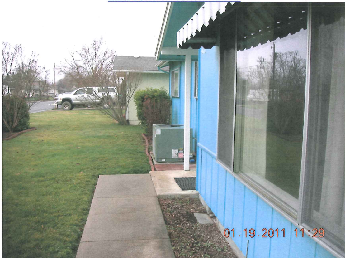
HEAT PUMP ON CONCRETE PAD
