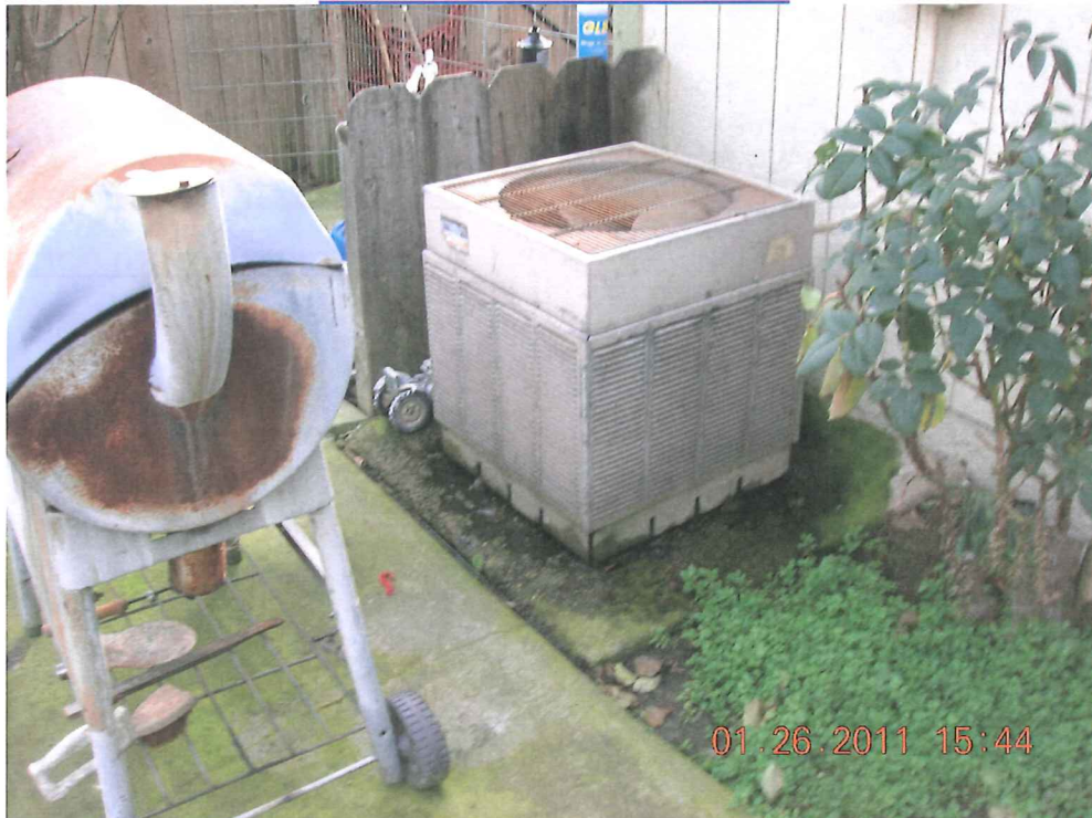
HEAT PUMP ON CONCRETE PAD
