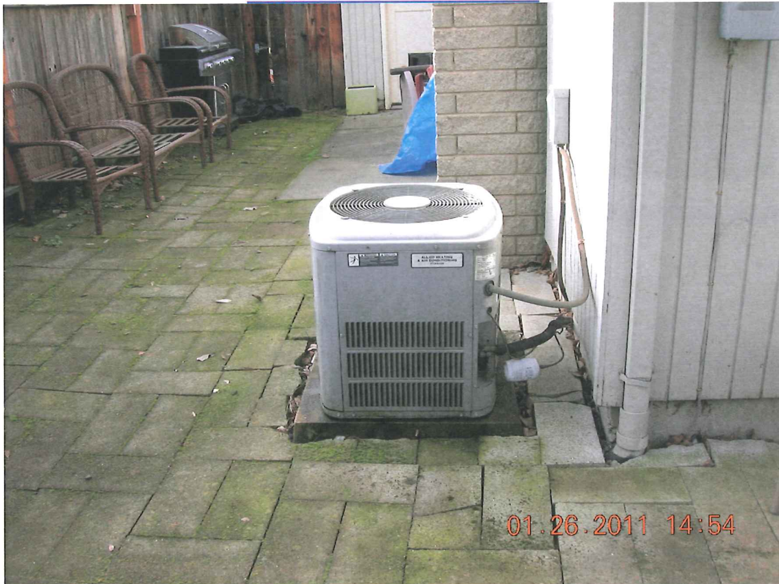
HEAT PUMP ON CONCRETE PAD
