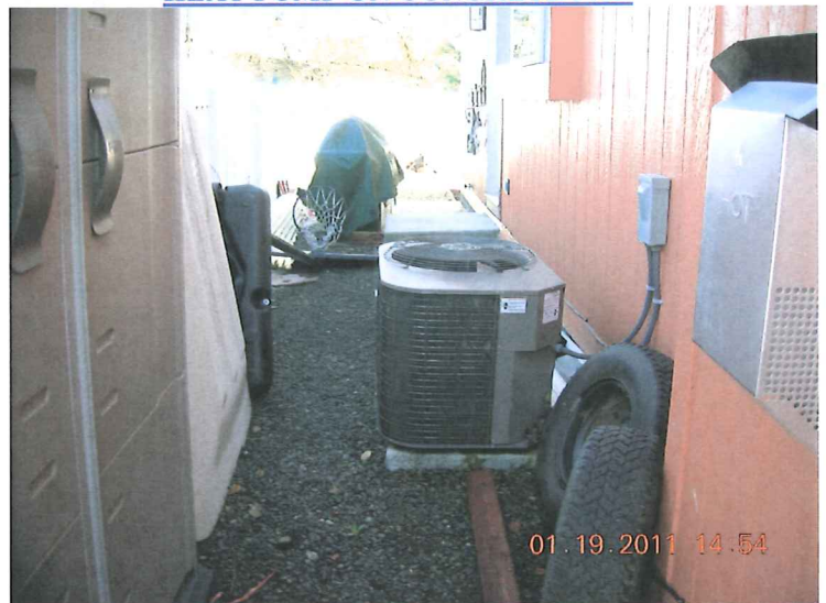
HEAT PUMP ON CONCRETE PAD
