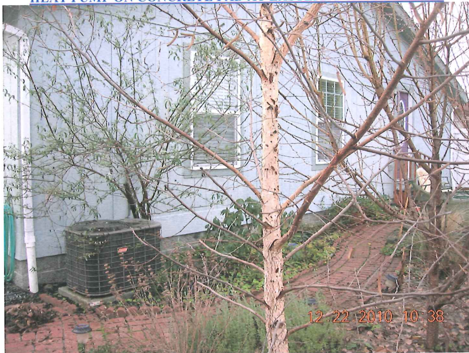
HEAT PUMP ON CONCRETE PAD AT EASTERLY SIDE OF HOME
