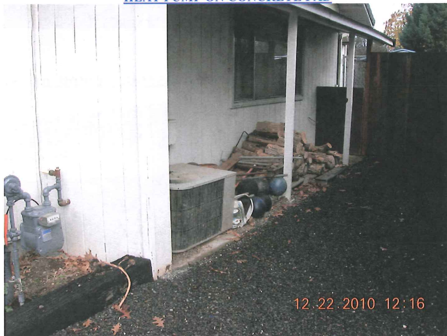
HEAT PUMP ON CONCRETE PAD
