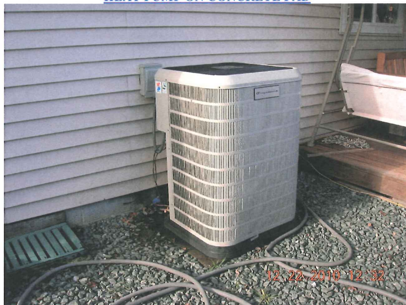
HEAT PUMP ON CONCRETE PAD
