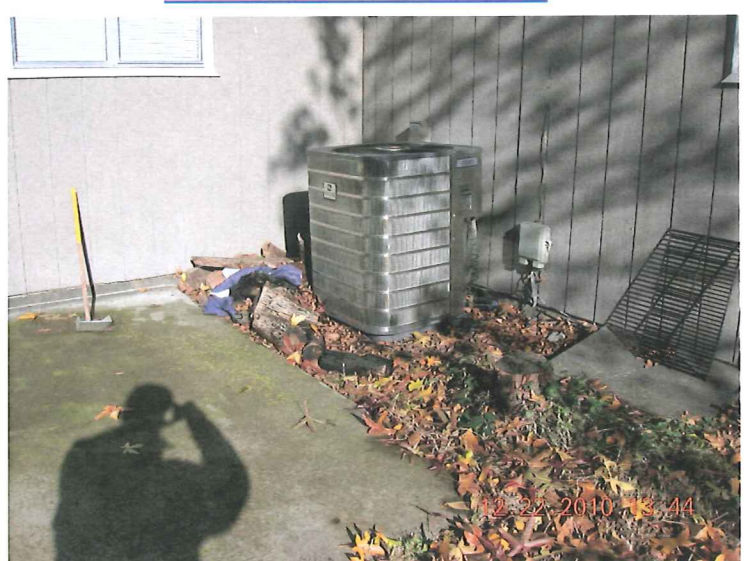
HEAT PUMP ON CONCRETE PAD
