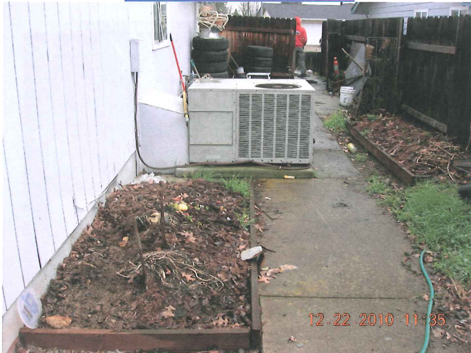
HEAT PUMP ON A CONCRETE PAD
