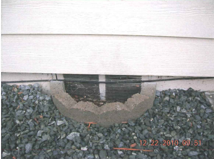
FOUNDATION VENT WITH LOUVERED COVER (1)
