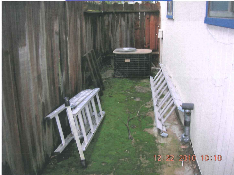
HEAT PUMP ON CONCRETE PAD
