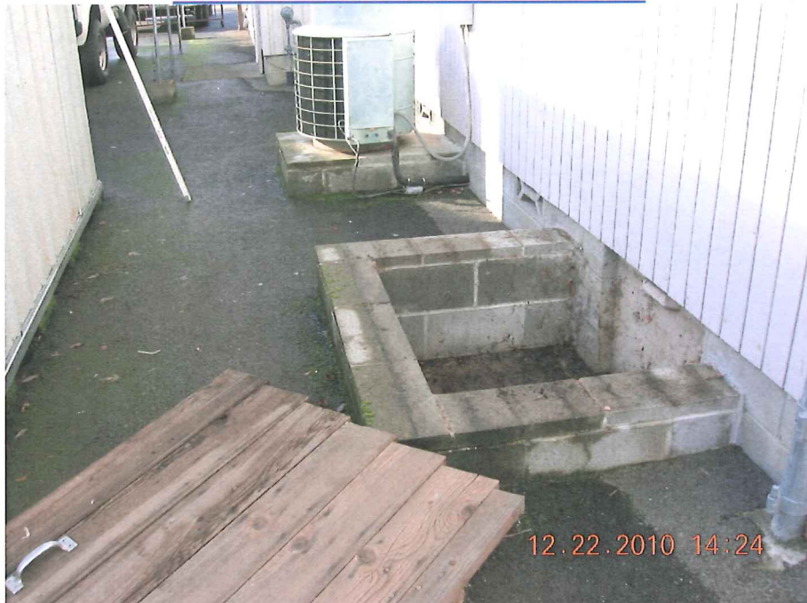
CRAWLSPACE ACCESS AND HEAT PUMP
