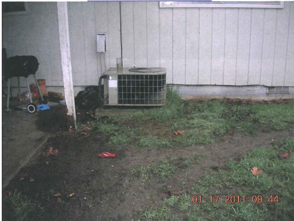
HEAT PUMP ON CONCRETE PAD
