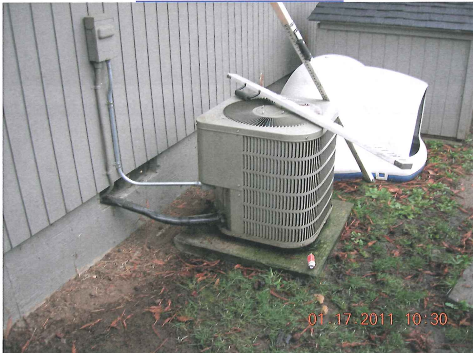
HEAT PUMP ON CONCRETE PAD
