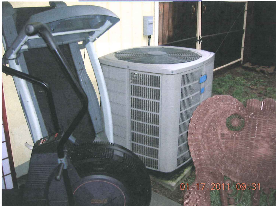
HEAT PUMP ON CONCRETE PAD
