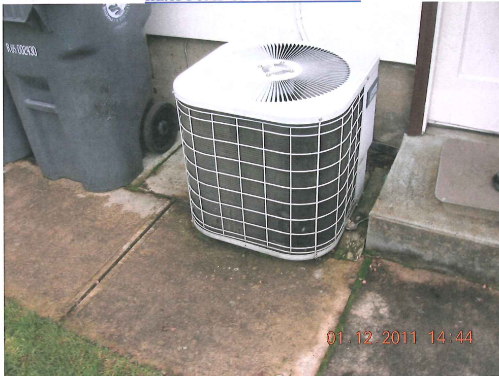
HEAT PUMP ON CONCRETE PAD
