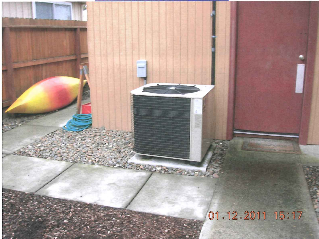
HEAT PUMP ON CONCRETE PAD
